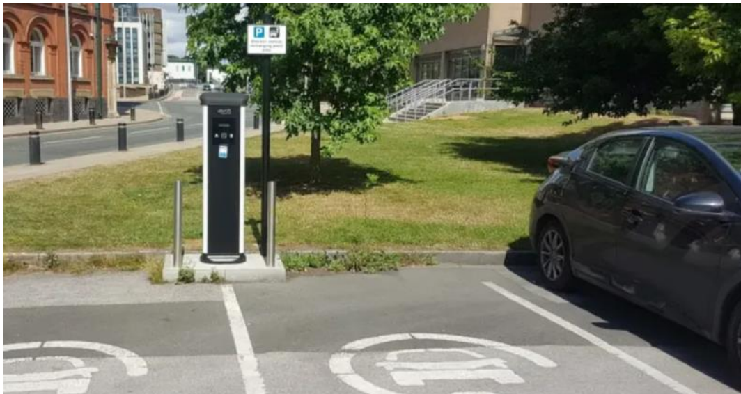
An example of a car park charger (picture from Hull City Council)
