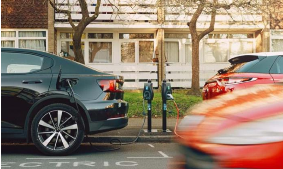
An example of an on-street residential parking charger (picture from West Sussex County Council)
